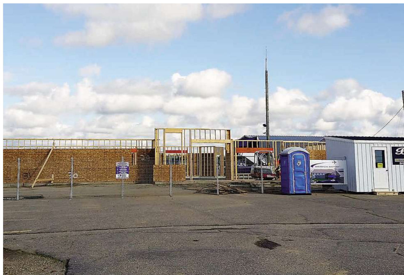
A look at the construction of the new Miramichi Airport terminal being built this week. PHOTO: KRIS MCDAVID/MIRAMICHI LEADER
