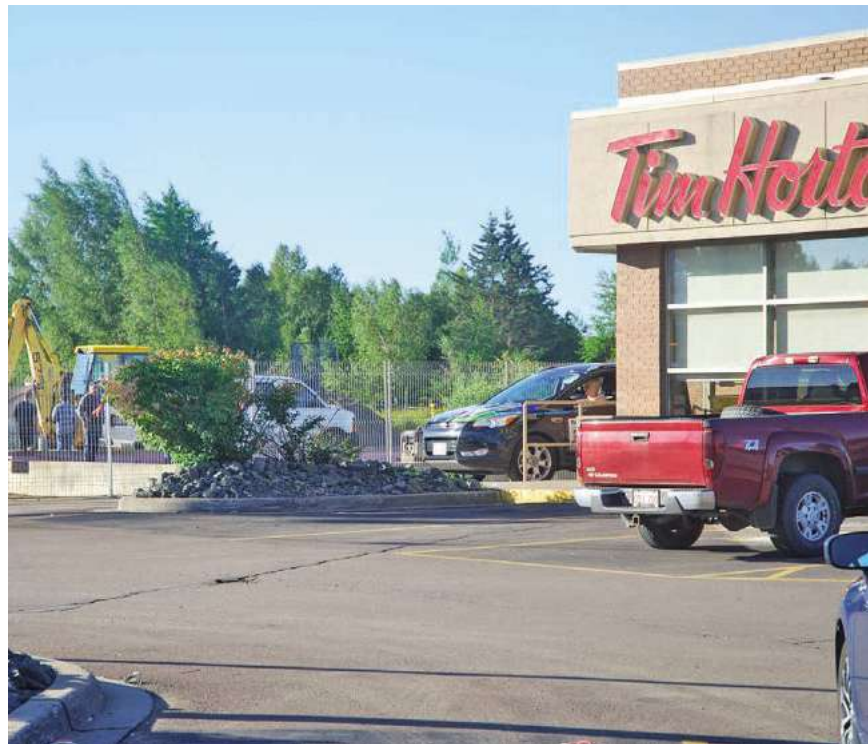
Construction work has begun on a new Tim Hortons in Miramichi, which will be adjacent to the current restaurant. PHOTO: LUKE CARROLL/MIRAMICHI LEADER
