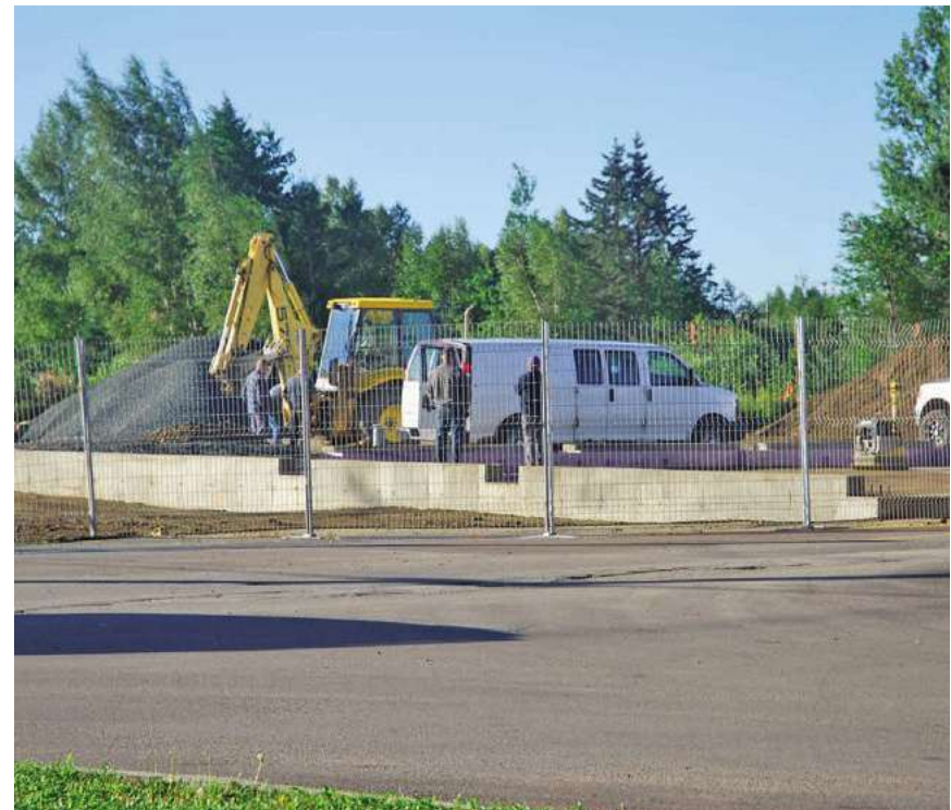
Workers can be seen on site at the new Tim Hortons location on King Street/Route 11. PHOTO: LUKE CARROLL/MIRAMICHI LEADER
