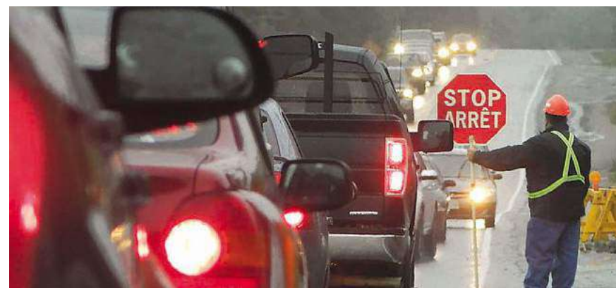
"Construction crews are working to make the highways safer for you. When you slow down, you make the workplace safer for them," says Gerard Adams, president and CEO of WorkSafe New Brunswick. PHOTO: MIRAMICHI LEADER ARCHIVES
