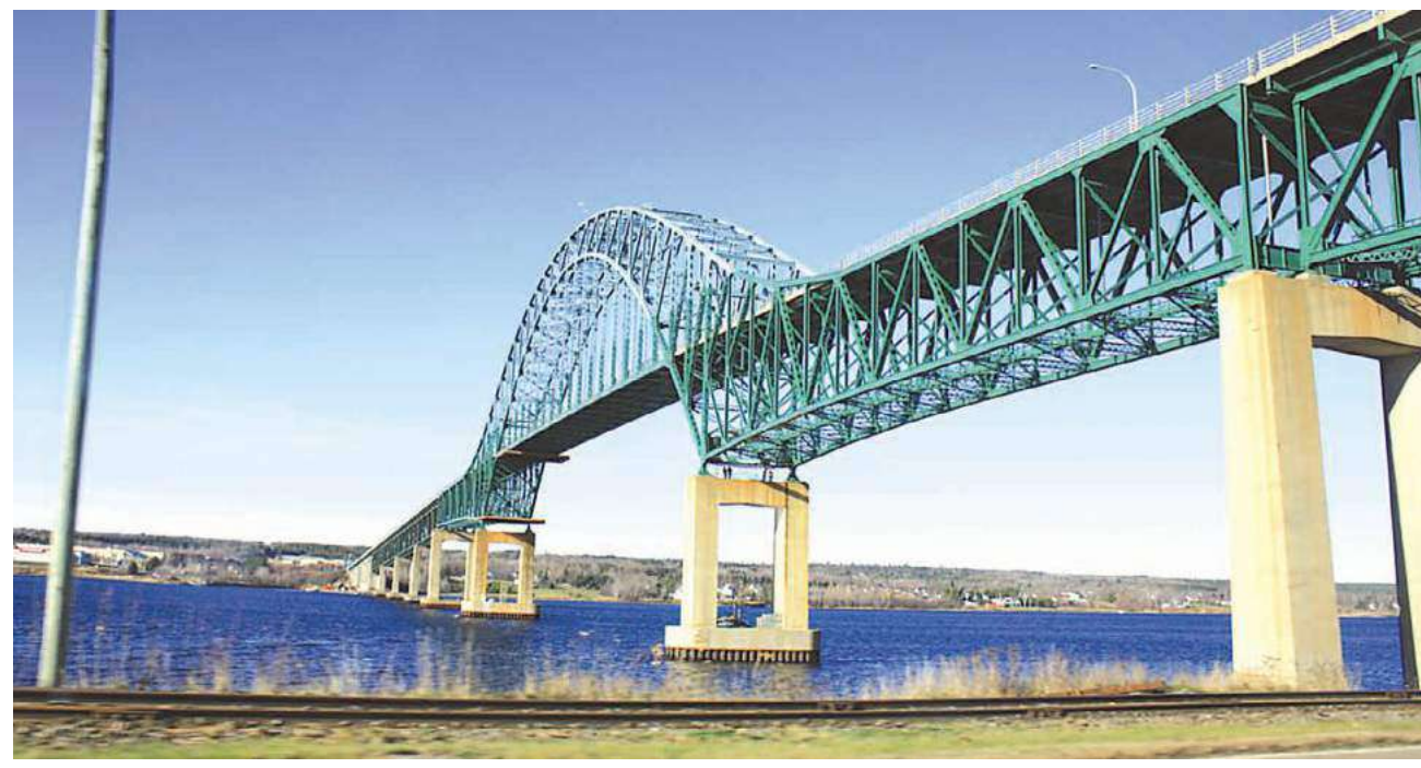
The federal and provincial governments are committing a combined total of $82.8 million to carry out further repairs to the Centennial Bridge in Miramichi. The work will be spread over nine years. PHOTO: MIRAMICHI LEADER ARCHIVE
